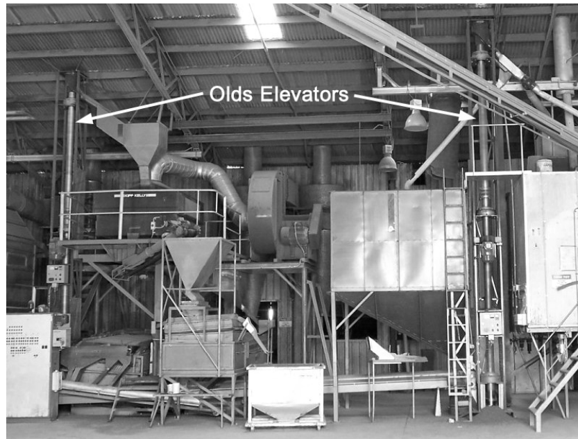
Figure 8 Two (2) × 150 mm N.B. Olds Elevators at BGA
