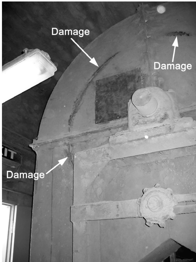
Figure 1 Examples of Damage to Bucket Elevator
