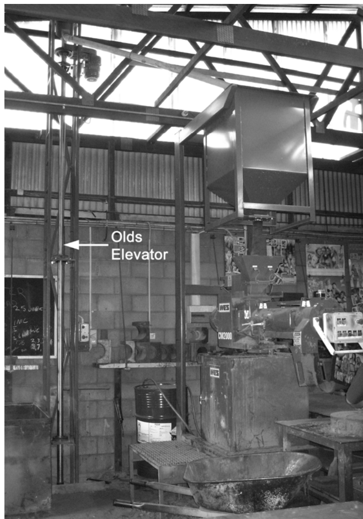
Figure 7 Original Olds Elevator installed in Olds Engineering Foundry
